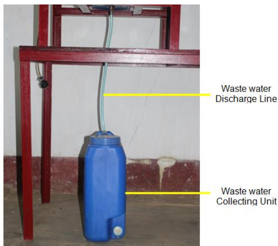
Figure 6: Waste water collecting unit
